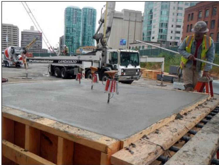
The sensor probes of RFID tags are embedded in a poured concrete, and the data is read remotely.
