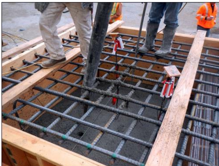
The collected data reduces the amount of time required for the cooling and hardening of concrete before the next slab can be poured
